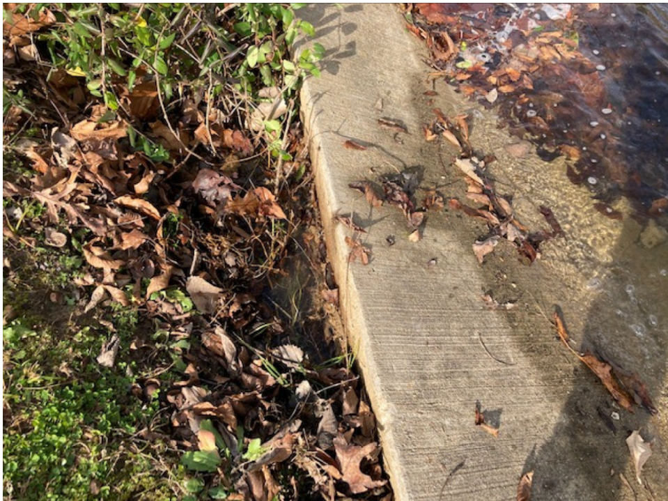
Photo #2: Depression Near Lower End of Spillway, 04 January 2021
