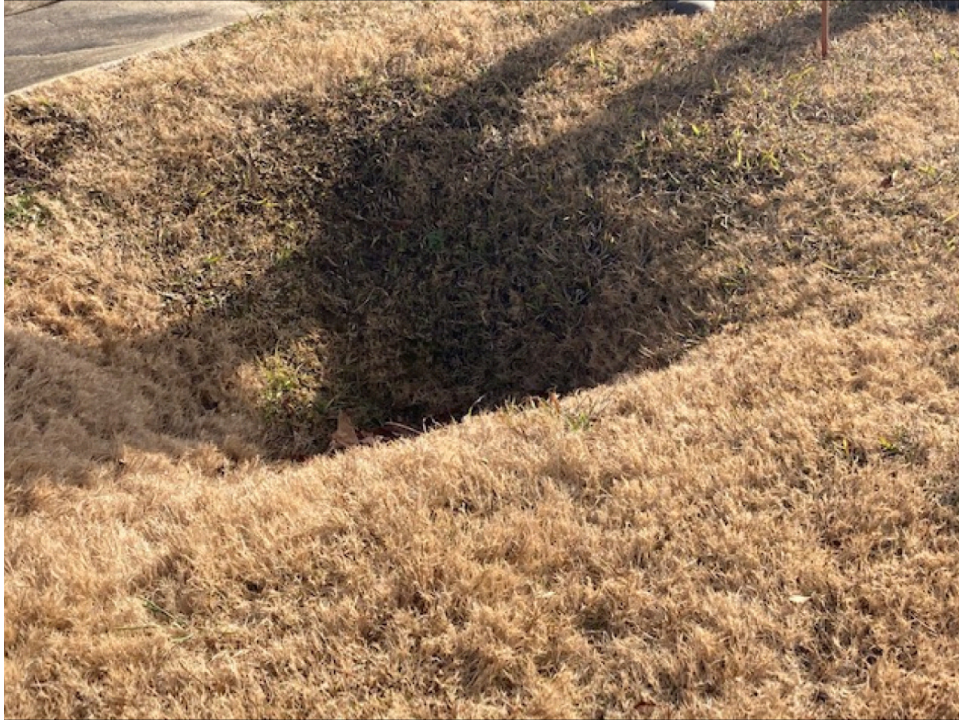
Photo #1: Sink Hole South of Upper End of Spillway, 04 January 2021
