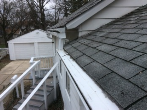
Gutters have guards, but still have debris - clogged
