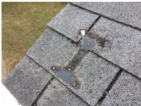
Dish mount removed, need holes plugged
