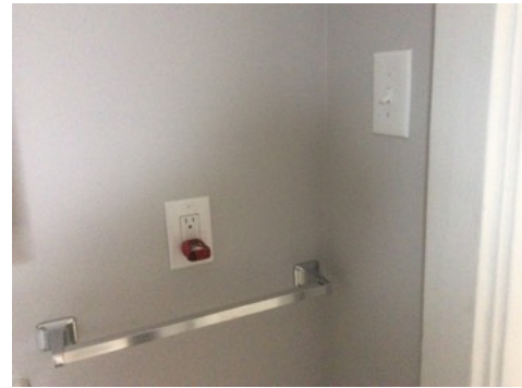
Power to outlet goes out when light is turned off
