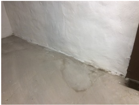
Water stains on floor suggests water seepage
