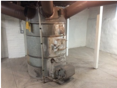
Very, very old heating unit - replace
