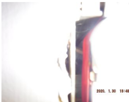
K&T wiring noted in home
