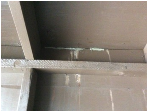
Leaking roof section
