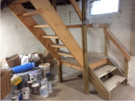
Steep with open slots at risers. No balusters
