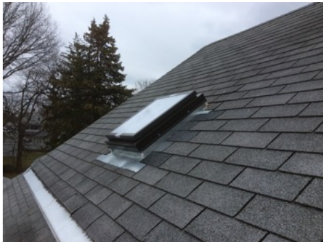
Appears to be recently installed
