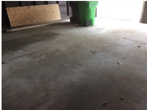
Typical cracking and settlement
