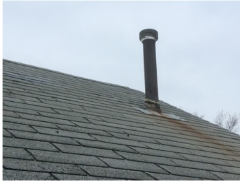
Waste vent pipe - should not have cap
