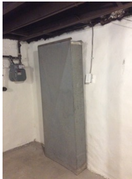
Return air drop - needs reconnected
