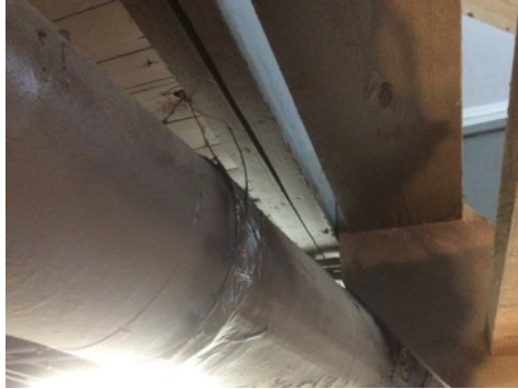
No brackets to hold stairs in place
