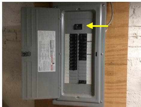
Main electrical disconnect - power shut off
