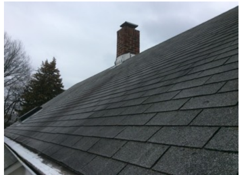
Older shingles - large gaps & lifting edges
