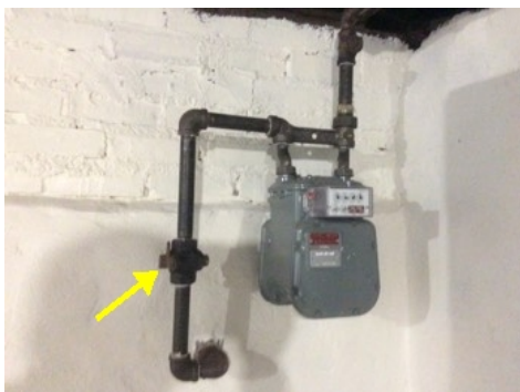
Main gas supply shut-off valve
