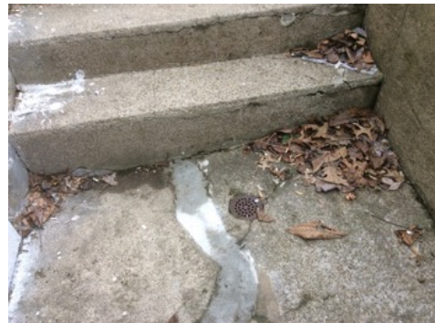
Keep area / drain clear of debris
