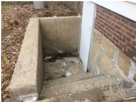
Rear steps, no handrail
