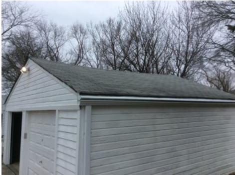
Aging shingles noted
