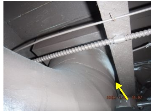
Possible asbestos material on ducts
