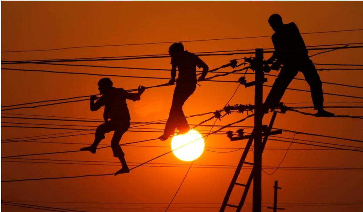
Figure 2.7 Electricity line workers in India. Safety standards in third world cultures differ markedly from those in first world nations due to differences in resources and possibly due to the difference in the value of life. 28
