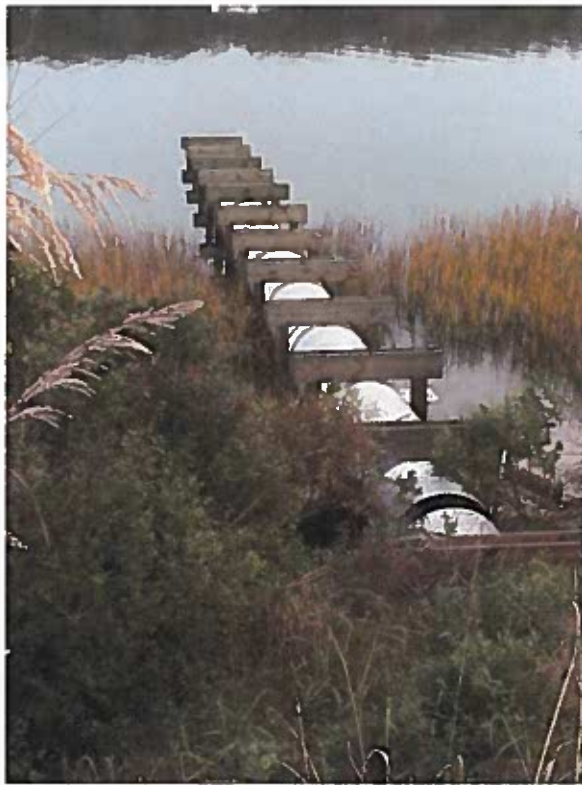
Disposal Area Discharge Pipe
