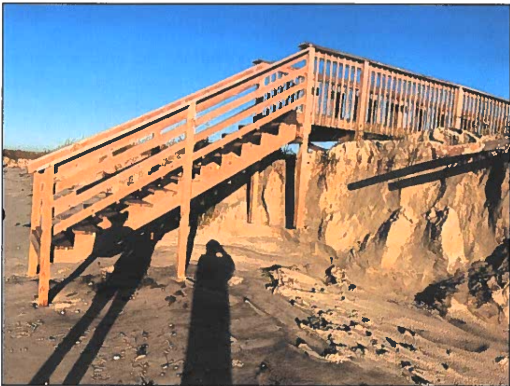
Figure 2-31. West End Dune Erosion and Vegetation Loss
