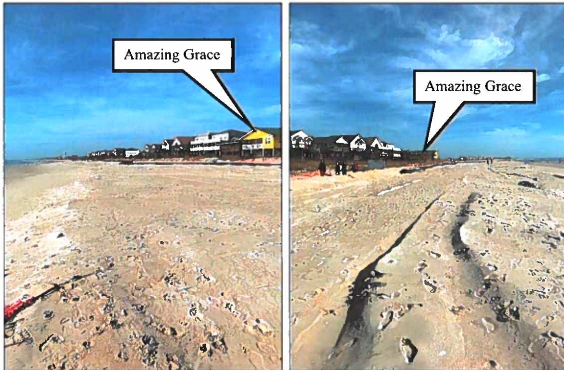
Figure 2-24 (a). Photograph in East End Taken During 2020 LWFIX Construction. (Holden Beach Town Newsletter)
