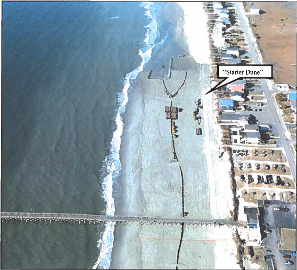
Figure 2-7. Aerial Photograph during Central Reach Construction West of Pier, Approximately Station 180+00 (Weeks Marine/Aerophoto Photo 2/22/17).
