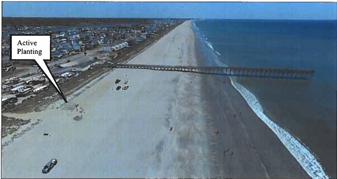
Figure 2-9 (D). Aerial Photograph Take From ~Station 180+00 Following CRR Construction During Active Planting Efforts Near Pier (ATM photo taken 04/28/2022).
