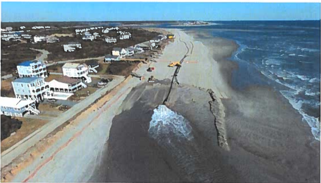
Figure 2-16. Holden Beach POA Aerial Photograph taken during 2017 Eastern Reach Project Construction (pumping just west of Station 30+00).
