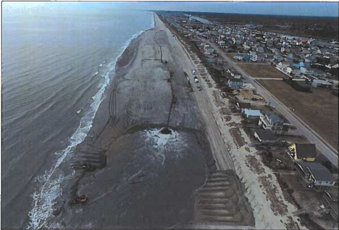
Figure 2-9 (A). Aerial Photograph During CRR Construction, Photo Taken Near East Taper, ~Station 40+00, Looking West (ATM Drone Photo 01/20/22).
