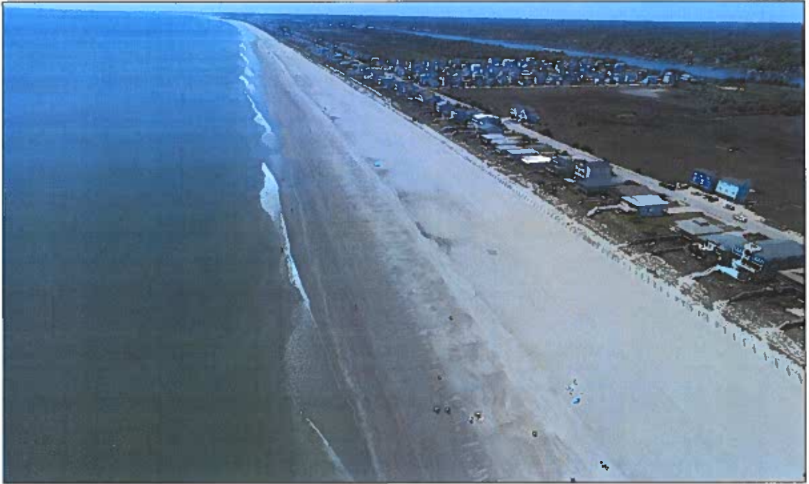
Figure 2-9 (B). CRR Post-Construction Aerial Photograph Taken Near Pier looking west (ATM photo taken 04/28/2022).
