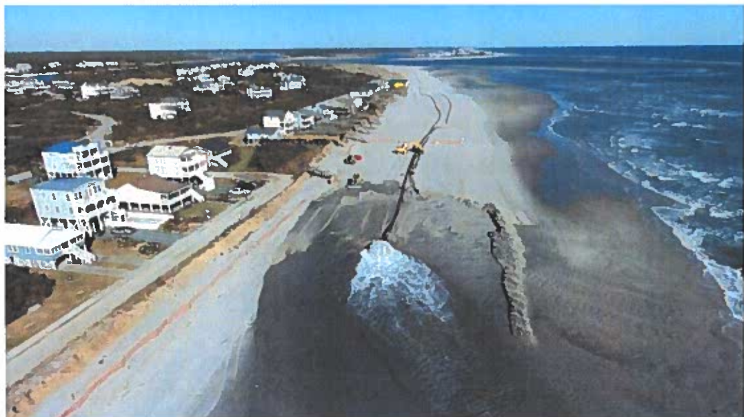
Figure 2-16. Holden Beach POA Aerial Photograph taken during 2017 Eastern Reach Project Construction (pumping just west of Station 30+00).
