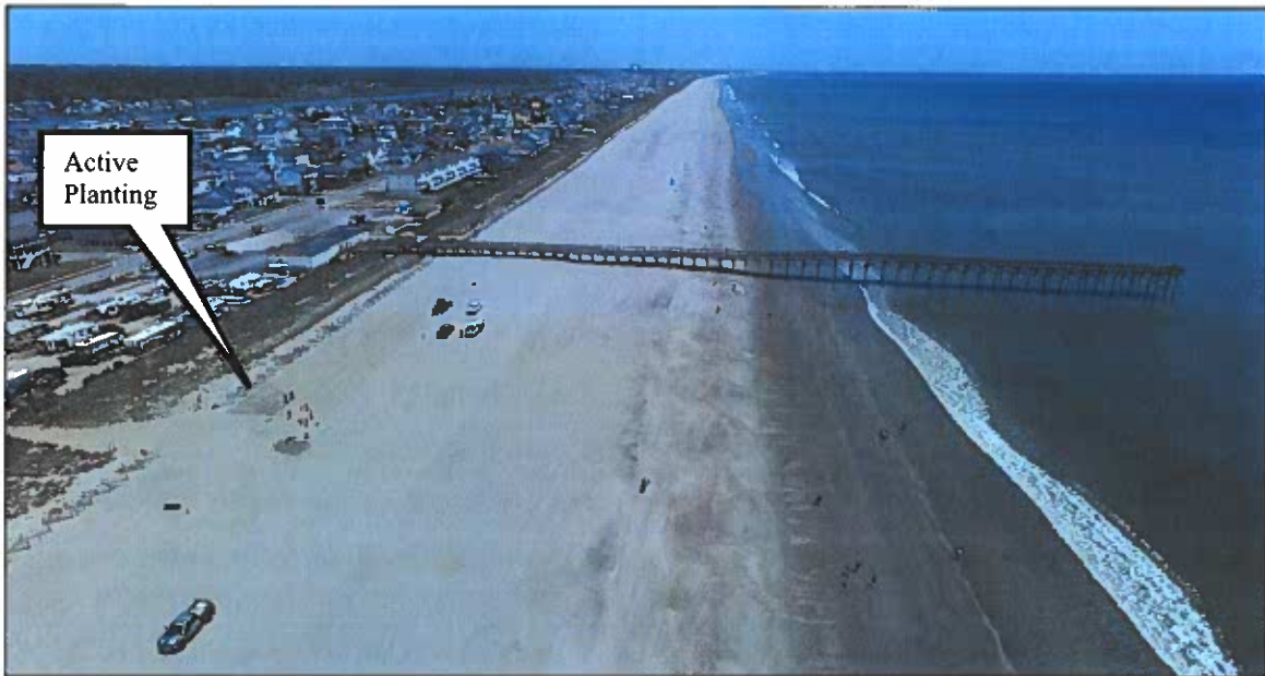
Figure 2-7 (D). Aerial Photograph Take From ~Station 180+00 Following CRR Construction During Active Planting Efforts Near Pier (ATM photo taken 04/28/2022).
