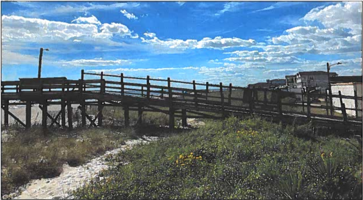
Figure 2-11 (F). October 2021 photo. New plantings along the landward dune (left hand side of photo) have suffered some damage (likely from Isaias in August 2020), but dunes are overall healthy.
