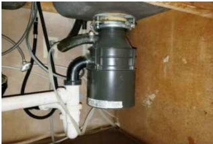
Garbage disposal was functional
