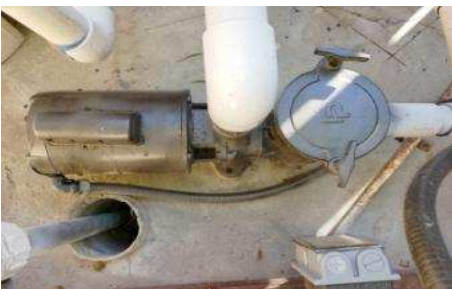
Pump was functional
