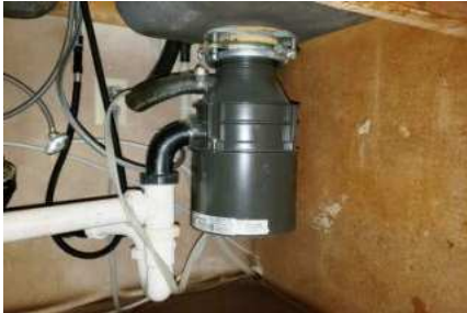
Garbage disposal was functional
