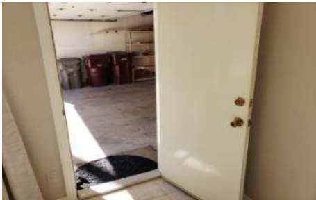
Fire door closure was inoperable
