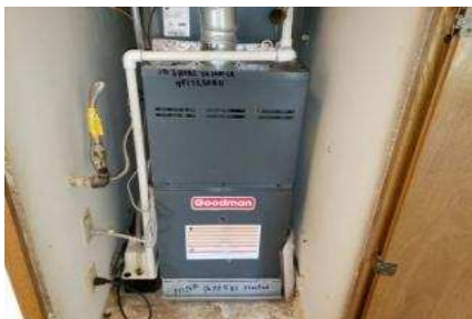
Furnace was functional
