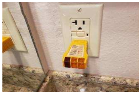
GFCI outlet not responding correctly
