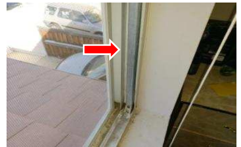
Window balancers were damaged
