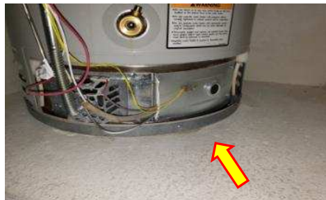
Missing drain pan
