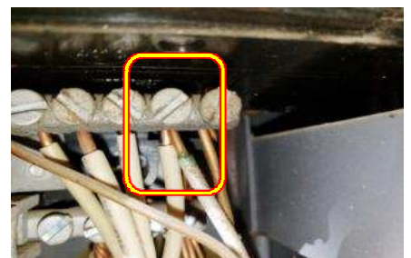
Neutral (white) wires were doubled or bundled together
