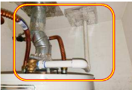
TPR pipe improper/runs uphill
