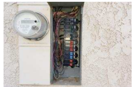
View inside main electrical service panel
