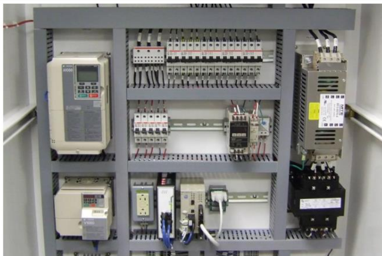
Panel de control industrial UL508A
