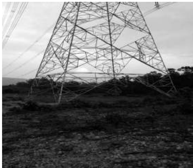
Photo 1: Tower of OGPTL near Sana Rampia Village
