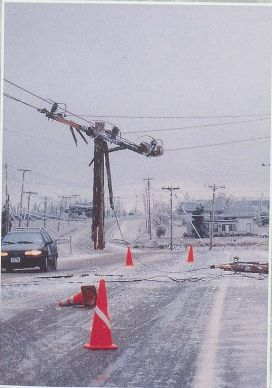
This pole snapped over Rt. 12E in Chaumont, New York.
