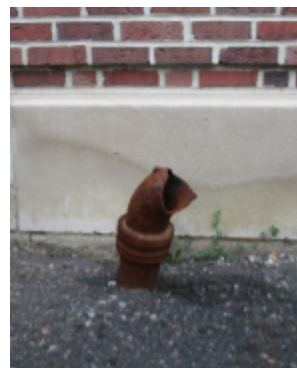
Photo 129 Location: West Facade Description: P trap from roof drains discharging at west side. Courtesy of Bob Marquardt
