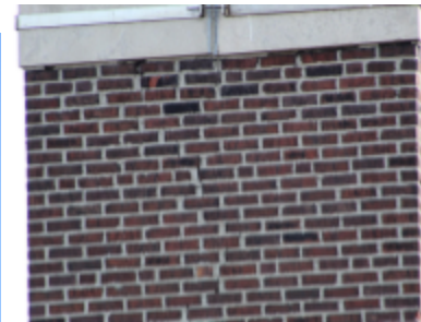
Photo 123 Location: West side of chimney taken from Backus roof. Description: Hairline cracks in mortar joints leading down from joint at limestone cap. Courtesy of Bob Marquardt.
