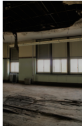
Photo 14 Location: Room 218 Description: Damage to wood floor in room 218. Courtesy of Citizens for Backus/AB
