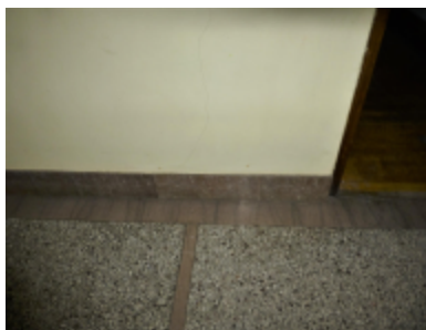
Photo 16 Location: Room 126 Description: Terrazzo corridor flooring with marble dividing strips and marble base.
