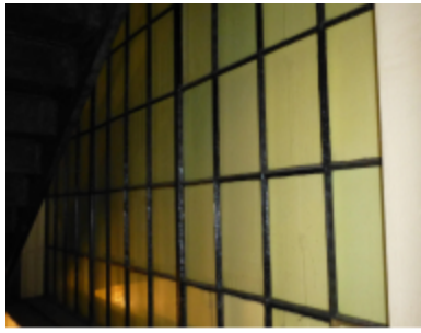
Photo 7 Location: west stair, corridor 25 Description: Original metal frame window at west stairwell as seen from inside.
