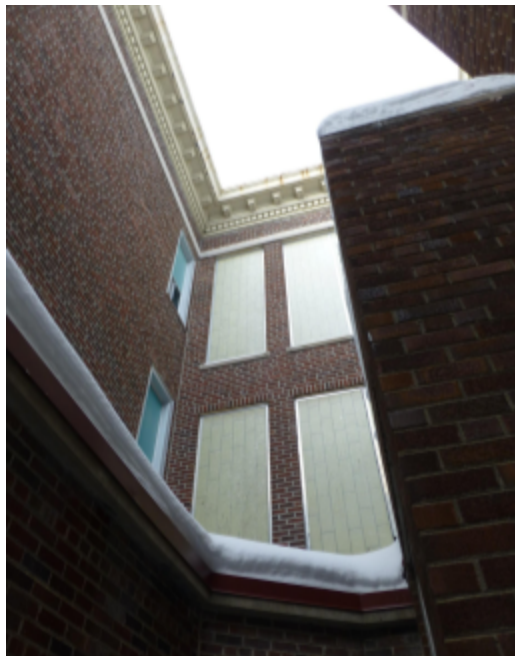
Photo 113 Location: southwest elevation Description: corner of southwest wing and west stair showing types of non-historic windows.
