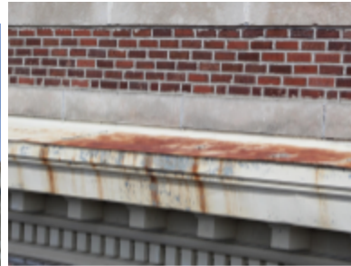
Photo 119 Location: South cornice Description: Rusting and staining on top of sheet metal cornice, typical. Courtesy of Bob Marquardt
