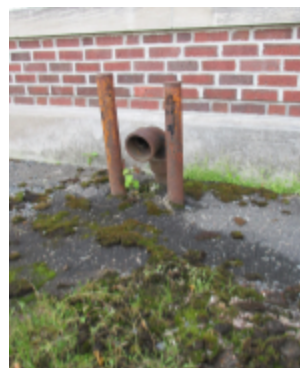
Photo 128 Location: North Facade Description: P trap from roof drain discharging at north side. Courtesy of Bob Marquardt
