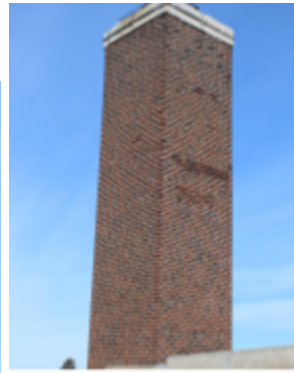
Photo 121 Location: SE corner taken from roof of Backus building. Description: View of chimney showing location and extents of damage on south/east sides. Courtesy of Bob Marquardt
