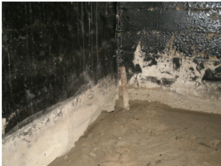
Photo 117 Location: Crawl space Description: wet soil in basement crawl space. Courtesy of Bob Marquardt
