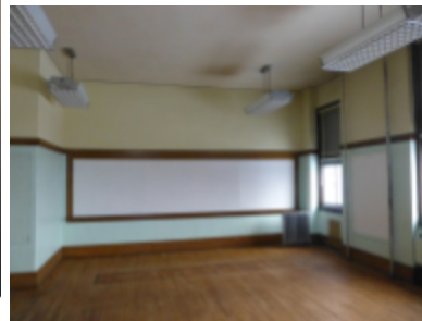
Photo 24 Location: Room 225 Description: Typical fluorescent style lighting fixtures in classrooms.
