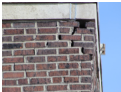
Photo 122 Location: Southeast corner of chimney taken from Backus roof. Description: Failed mortar joints and shifting of brick near limestone cap. Courtesy of Bob Marquardt.
