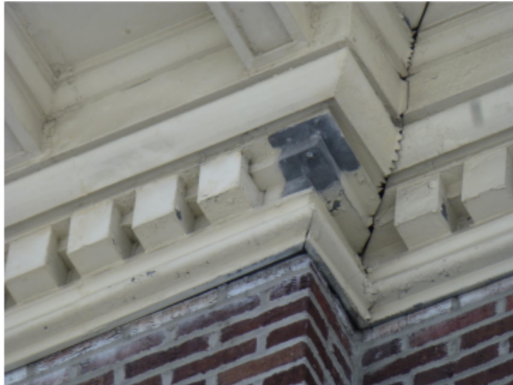
Photo 103 Location: east elevation Description: Missing dentil at corner of cornice. Slight efflorescence below cornice at multiple locations.
