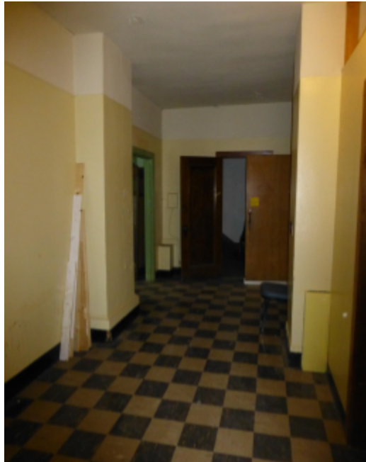
Photo 51 Location: Room 28 Description: Modifications to room 28. Non-historic door at right currently used to seal off these rooms from main corridor.
