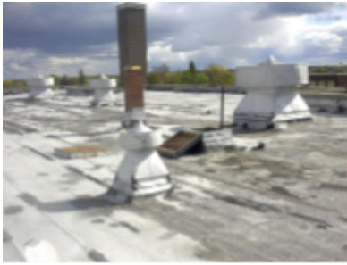
Photo 125 Location: Roof looking east Description: Roof with ventilators prior to re-roofing. Courtesy of Citizens for Backus/AB
