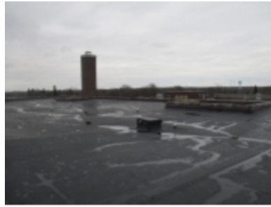
Photo 126 Location: Roof looking east Description: Roof after replacement. Appears to drain properly. Courtesy of Citizens for Backus/AB
