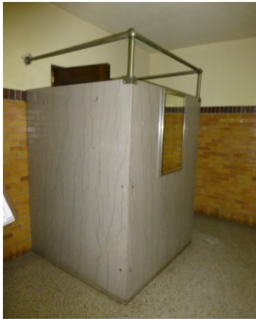
Photo 68 Location: Room 23 Description: Marble partition at entry to Women's restroom. Note Glazed brick wainscoting.
