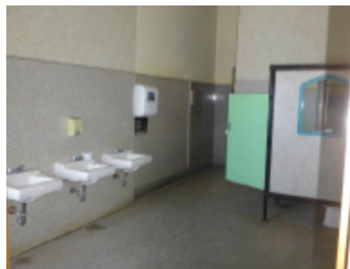
Photo 28 Location: Room 213 Description: Replacement fixtures in men's restroom on level 2. Replacement plywood door and laminate on partitions visible.
