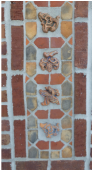
Photo 107 Location: north elevation Description: Detail of glazed terra cotta reliefs and decorative brickwork around north entry doors.
