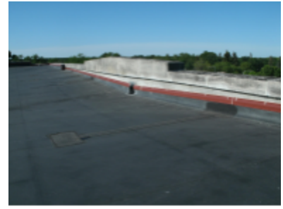
Photo 127 Location: Roof Description: Parapet walls and flashings after roof replacement. Courtesy of Bob Marquardt
