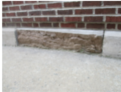
Photo 124 Location: Foundation Description: Deteriorated limestone at water table course. Courtesy of Bob Marquardt
