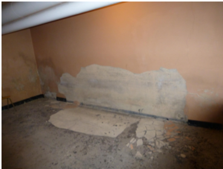
Photo 43 Location: Room B15 Description: Plaster separating from concrete wall in basement.
