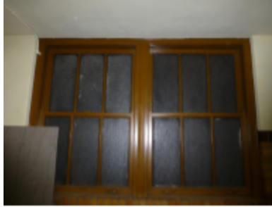
Photo 8 Location: Room 23, Women's restroom Description: Remaining historic wood windows in women's restroom on ground level covered over on exterior by Backus addition.
