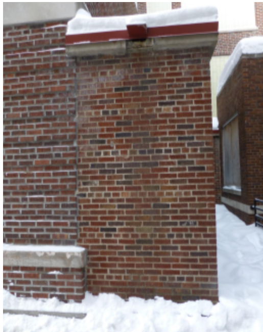
Photo 111 Location: southwest elevation Description: hole beneath replacement scupper on addition to building over tunnel stairs.
