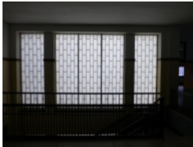
Photo 10 Location: Room 222, west stair Description: Typical fiberglass insulated replacement windows at stairwells.
