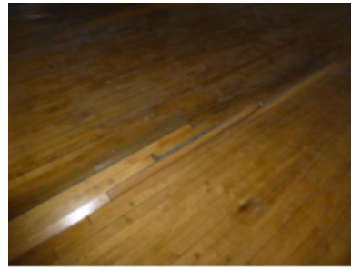
Photo 13 Location: Room 207 Description: Example of Buckling of wood flooring.
