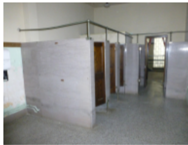
Photo 30 Location: Room 204 Description: Original marble stall partitions in women's restroom 204 shown with their original wood doors.
