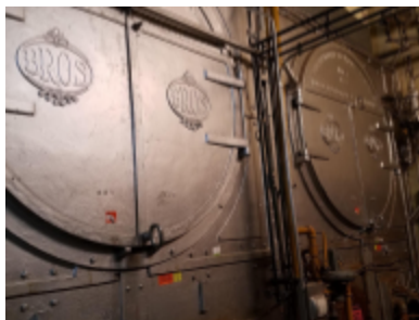
Photo 31 Location: Room B03 Description: The buildings two original steam boilers which have been recently rebuilt and currently serve to heat the Backus Building.
