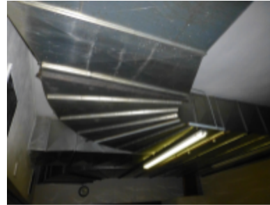
Photo 34 Location: Room 124 Description: Ductwork from central air handler at ceiling of level 1 installed when the Backus building was built.
