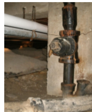
Photo 130 Location: Basement crawl space Description: Roof drain with seasonal changeover valve. Courtesy of Bob Marquardt
