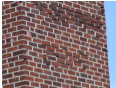
Photo 120 Location: Southeast corner of chimney taken from Backus roof. Description: Spawling face brick and deteriorated mortar joints on east side of chimney. Courtesy of Bob Marquardt.
