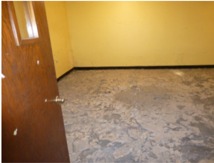
Photo 42 Location: Room B12 Description: peeling painted floor of room B12.
