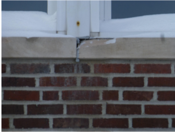
Photo 102 Location: east elevation Description: Damaged stone sill at level 1 window.
