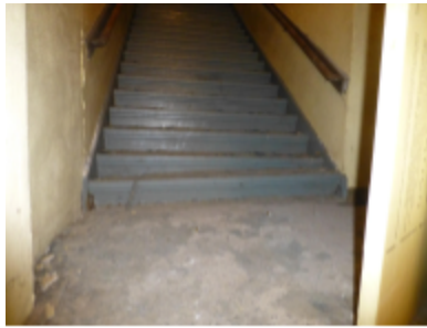
Photo 21 Location: Room B14, west basement stair Description: Stair treads damaged due to heaving.
