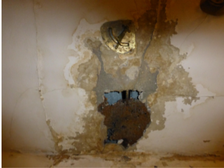
Photo 50 Location: Room 25 Description: Damage to corridor ceiling near damper valves.
