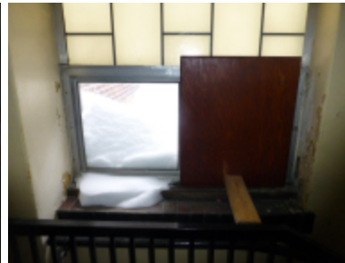
Photo 11 Location: Room 126, east stair Description: Failure at fiberglass insulated replacement windows at east stairwell.
