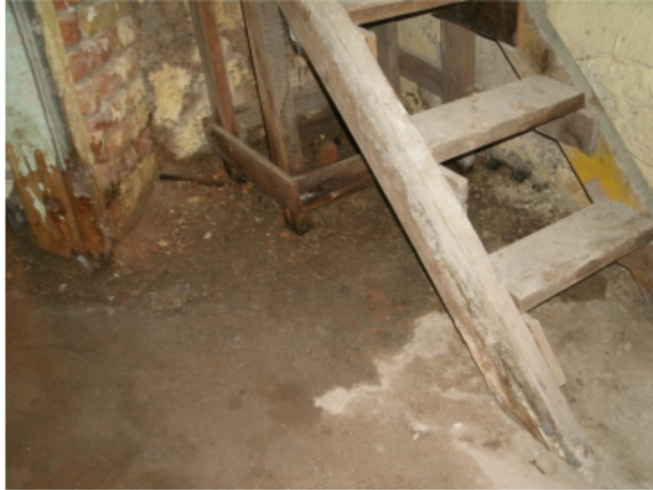
Photo 116 Location: B5 Description: wet basement floor near access to crawl space Courtesy of Bob Marquardt
