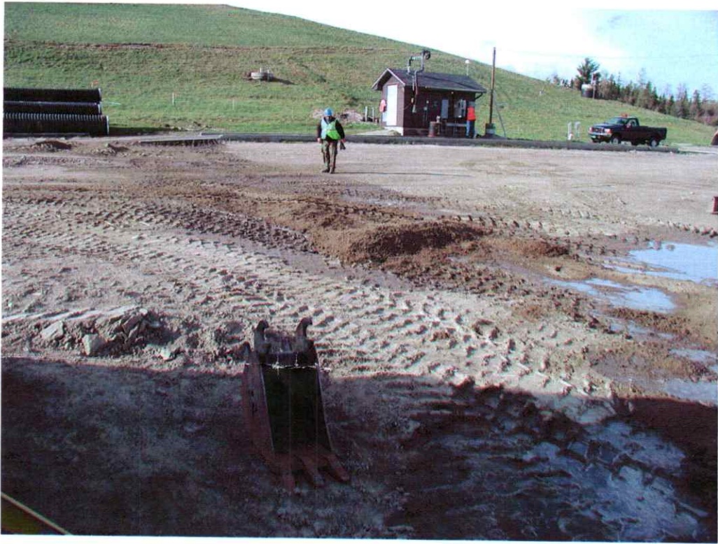
Leachate flow path across the perimeter road.
