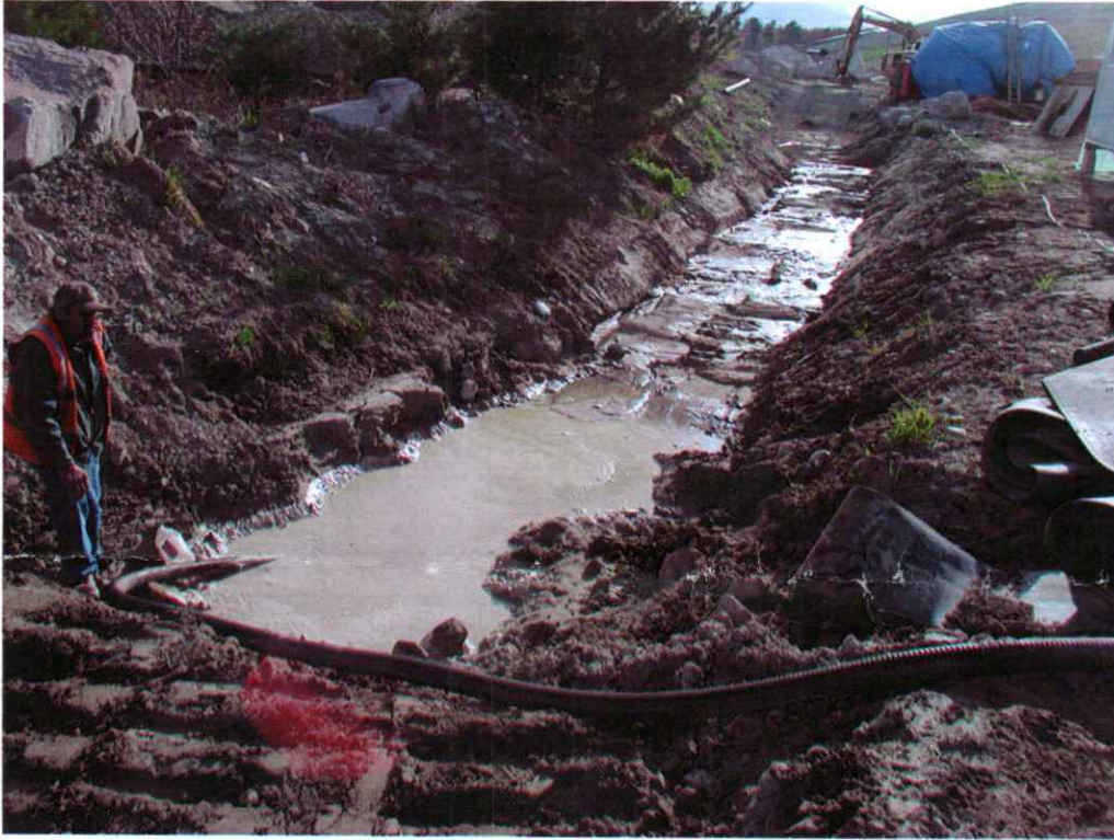
Loading tanker from contained leachate.
