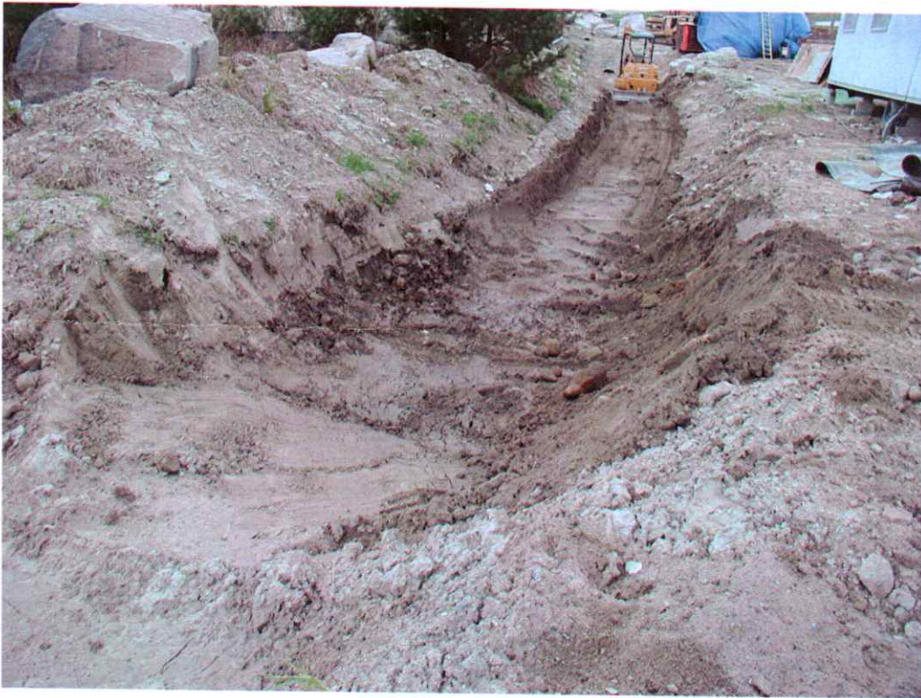
Storm water swale where leachate was contained as excavation was being completed.
