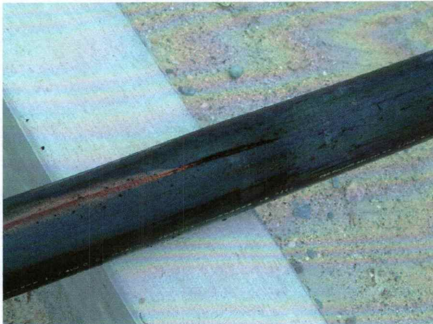
PHOTO #10 – Crack in vertical section of 2" containment pipe
