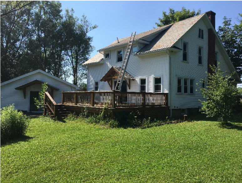
The high quality slate roof was professionally repaired. All cracked and dislodged slates were replaced and a new steel ridge installed.
