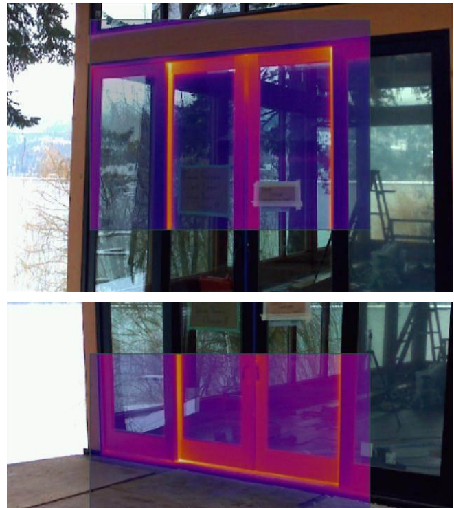
Fig.3.20 IR photo of a sliding glass door during depressurization (left) and pressurization (right), showing air leakage during pressurization around the door frame.
