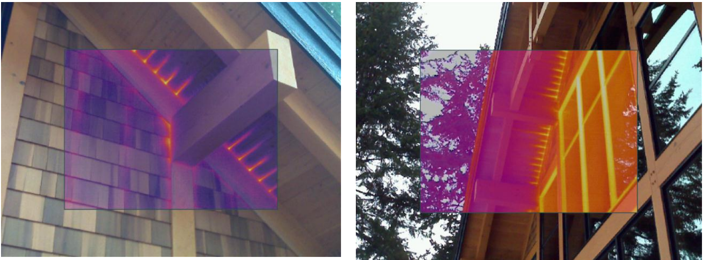
Fig.3.25 Air leakage at the roof to wall interface, both under pressurization.
