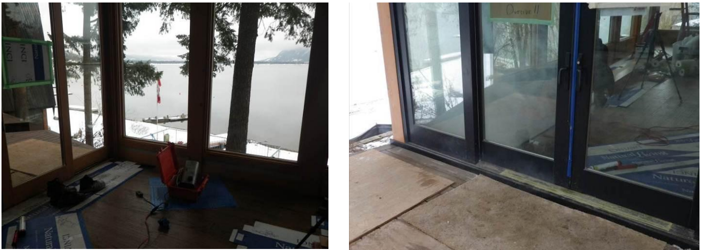
Fig.3.19 Theatrical fog machine used for smoke testing at a corner of the house (left) and smoke leakage observed around the sliding glass door (right) under depressurization.
