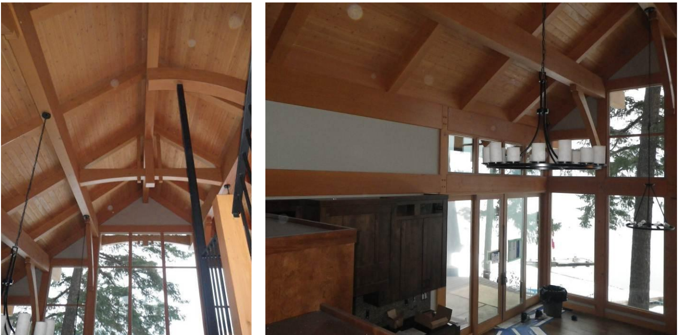
Fig.3.17 Cathedral ceiling and timber frame construction viewed from the inside of test house #3, Chase, BC.
