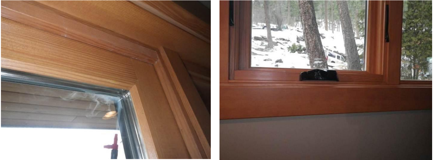
Fig.3.18 Smoke infiltration observed at sliding glass door between IGU and frame (left) and at operable window between sash and frame (right) under depressurization.
