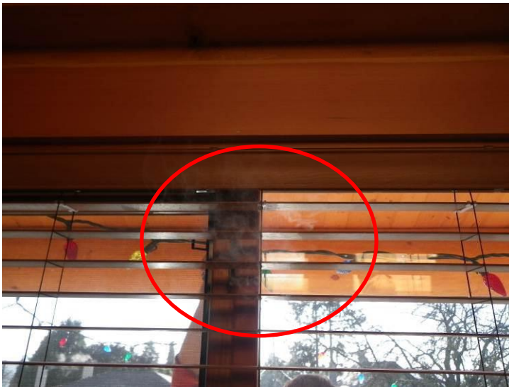
Fig.3.27 Smoke infiltration observed at corner joint during smoke testing from the interior under pressurization.
