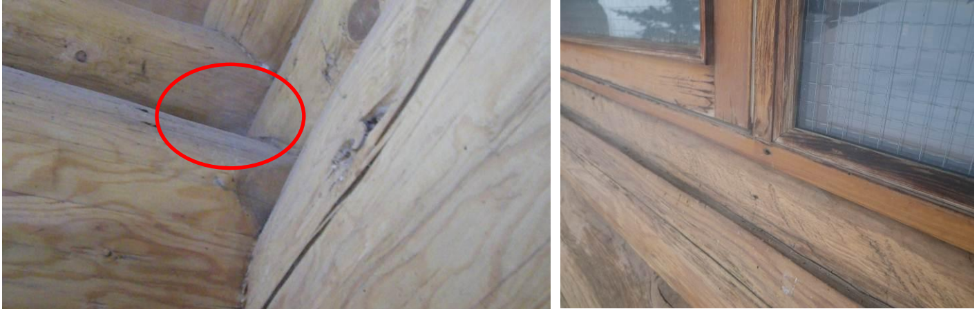
Fig.3.9 Smoke infiltration observed at corner joint (left) and around operable windows (right) during smoke testing from the interior under pressurization.
