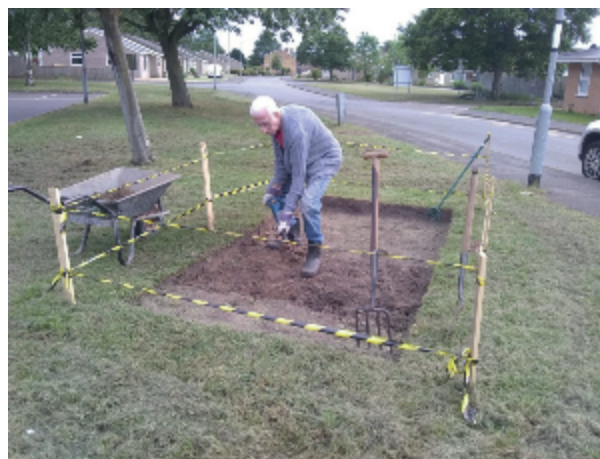
Above - Ted is pictured in the summer, helping to dig the footings for the installation.
