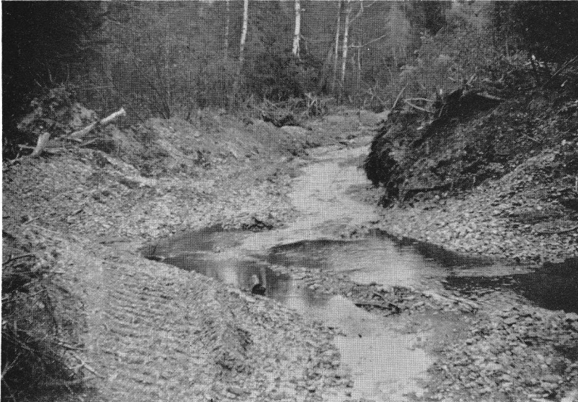
Figure 6. A section of Birch River bulldozed in 1954 in preparation for driving pulpwood.
