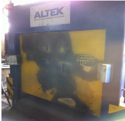
Figure 9 – Press Damaged by Thermiting Dross
