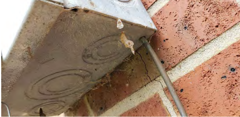
Laundry/Utility Room Electric Panel
