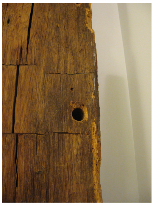
A detailed-view of one of the exposed, hard oak hand hewn beams in the house, showing a hole where a wooden peg ties together a cross-member.
