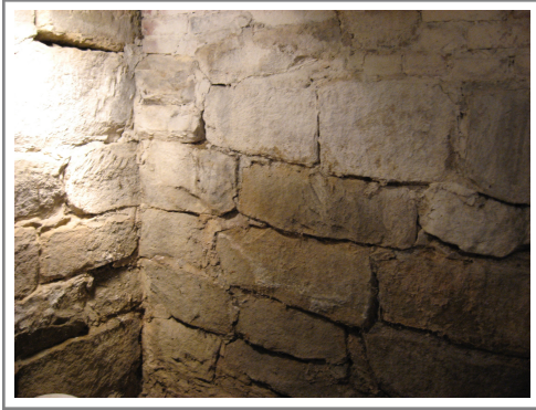
Hand cut blocks of sandstone comprise the Shupe house basement. These were quarried from a local outcropping of sandstone on Shupe's property.
