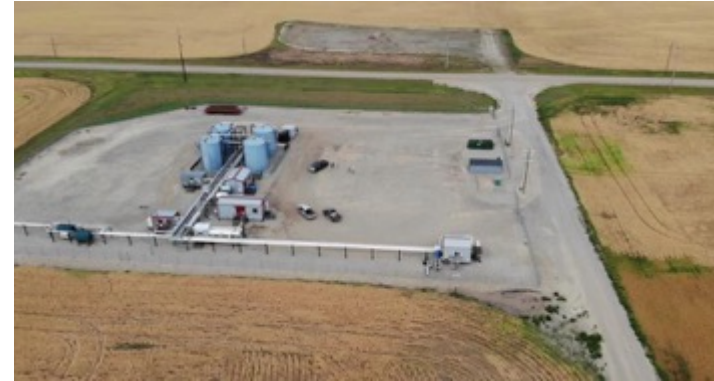
Vulcan 05-21 main multi-well facility equipped to handle 3 rd party processing
