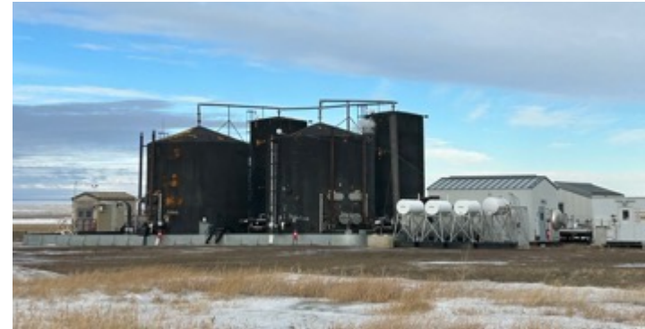
Murray Lake 7-36 main treating facility, consisting of separator, free water knockout, 5,000 bbls/d storage and water injection.
