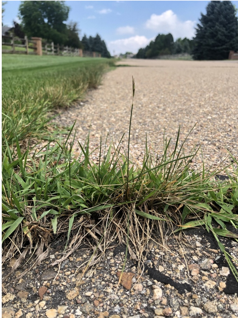
Cracks and weeds on Longview Drive
