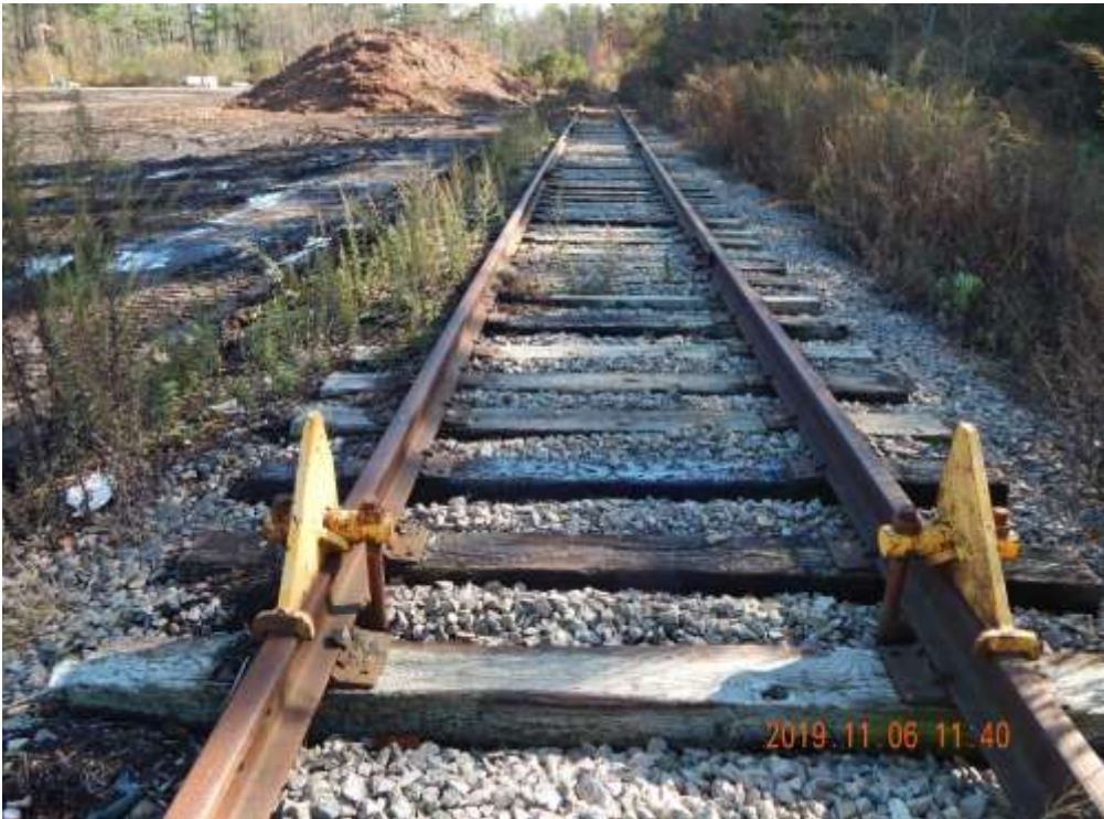
Fig. 10 Second potential Middleborough, Massachusetts transload location at end of spur (looking southeast)
