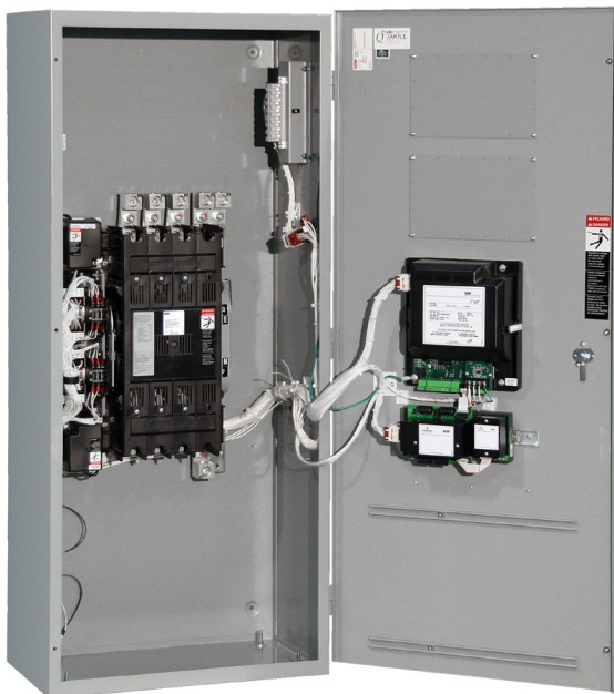
Fig. 16: ASCO 3ADTS/3NDTS 400 Amps Type 1 Enclosure
