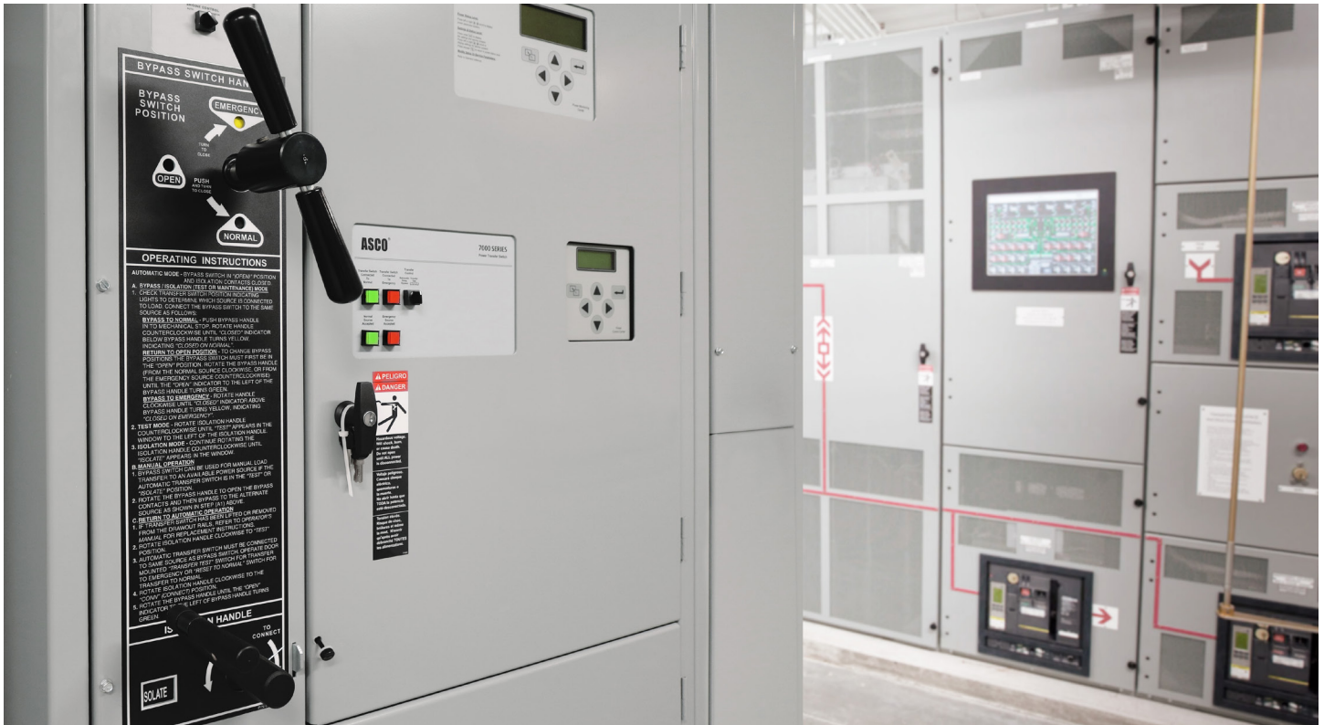
Figure 5 – Bypass and Isolation Handles
