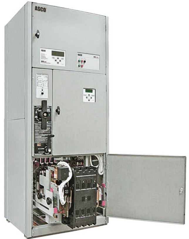
Figure 8: An ASCO J-Frame Isolation-Bypass Transfer Switch
