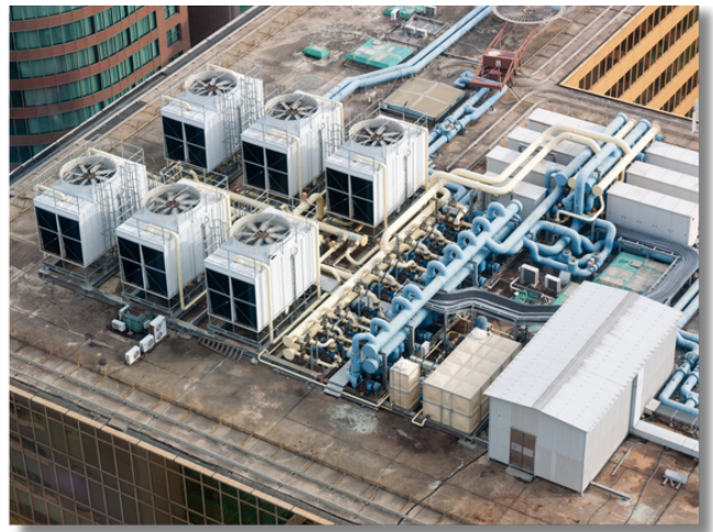
Six of the eight 450-ton cooling towers
