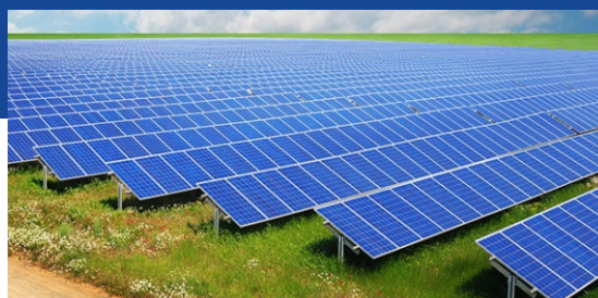
Solar Power & Energy Management
