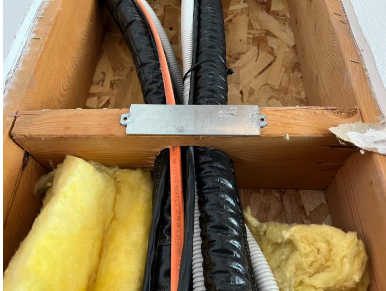
Close Up of Two-Line Sets with Panel Power (orange)
