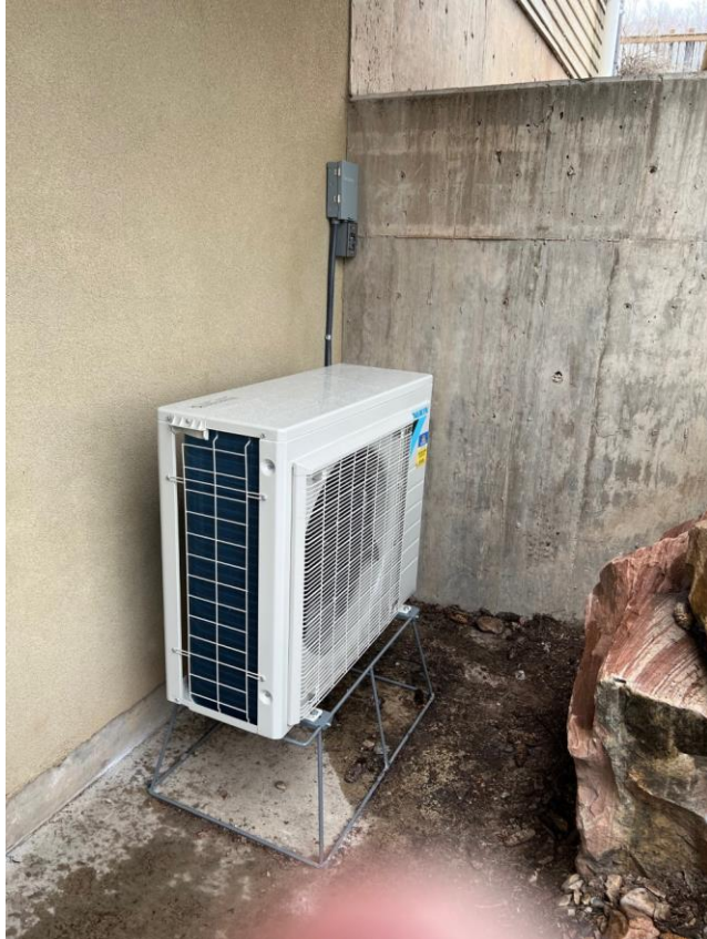
Outside Heat Exchanger)
