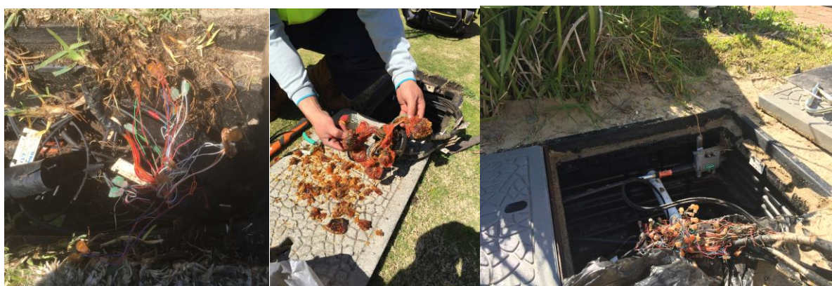
Figure 8.1 The current state of the copper telecommunications underground wires and the various attempts to stop copper from rusting (courtesy of 3A Kathy Telecommunications Pty Ltd)
