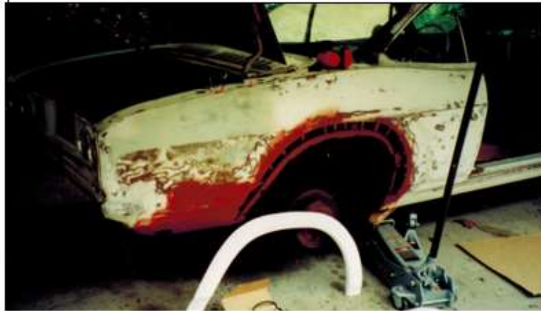
Wheel well area with rust cut away in 2001
