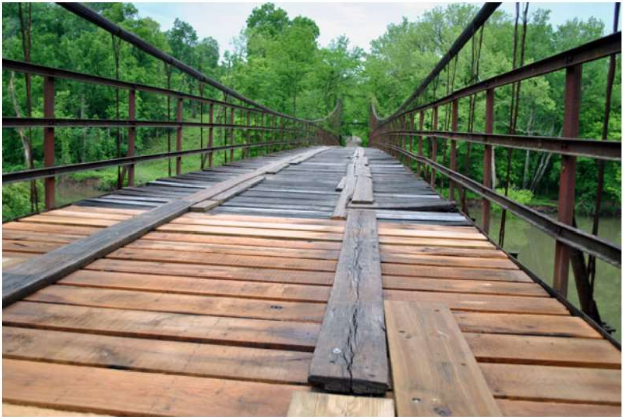
This May 2018 photo shows the Grand Auglaize Bridge, built in 1931 over the Grand Auglaize Creek, during a period when Miller County road crews were in the process of replacing floorboards. Photo by Allen Fennewald / News Tribune.
