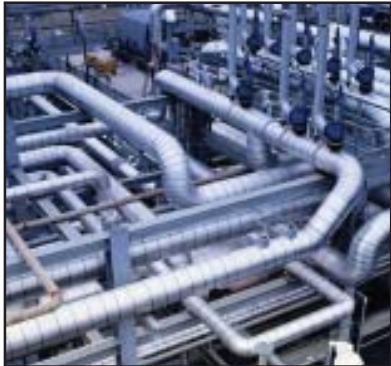
PGW delivers the natural gas from the city gate to the burner tip.
