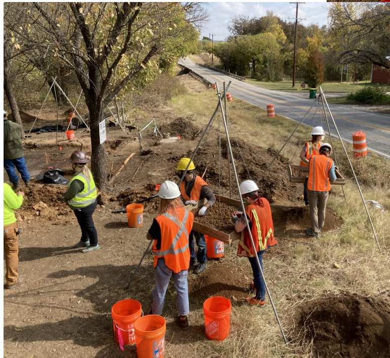
NTAS members screening at the Sartin Hotel Site the FM 455 in the background. As of May 1, 2021, TxDOT was given clearance to begin the road widening of FM 455 at the intersection
