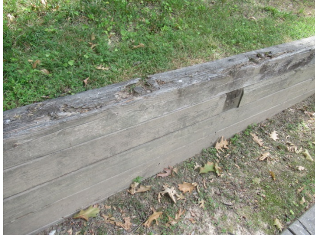
Timber retaining wall at Peter Roy Court overview – Note: wood rot
