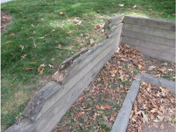
Timber retaining wall at Peter Roy Court overview – Note: wood rot and damage
