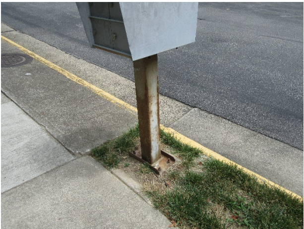
Mailbox station rust – Note: original station
