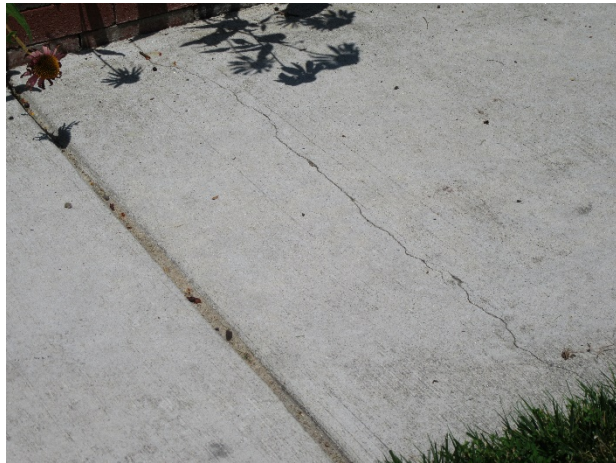
Isolated concrete sidewalk crack
