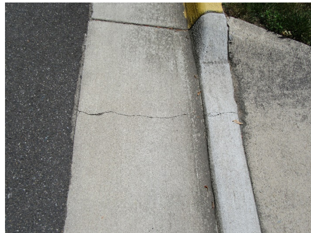
Cracked concrete curb and gutter
