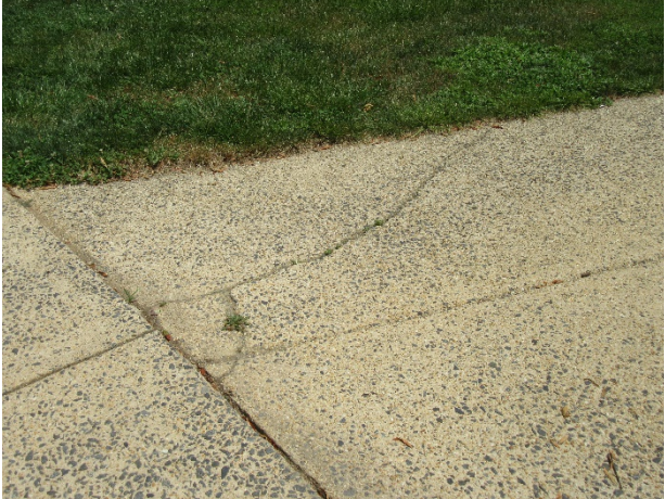
Concrete sidewalk crack
