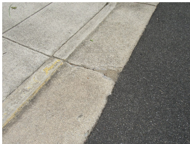
Minor spalled concrete gutter
