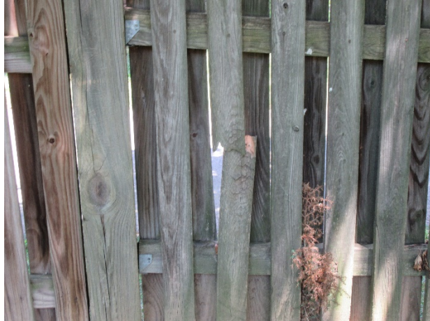
Damage to wood fence
