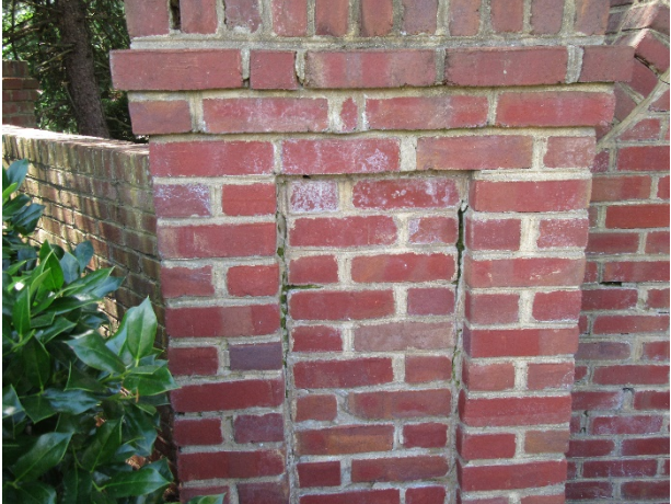
Mortar deterioration and efflorescence
