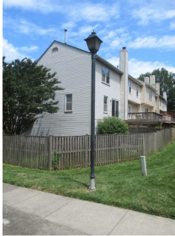
Light pole and fixture overview – Note: finish deterioration
