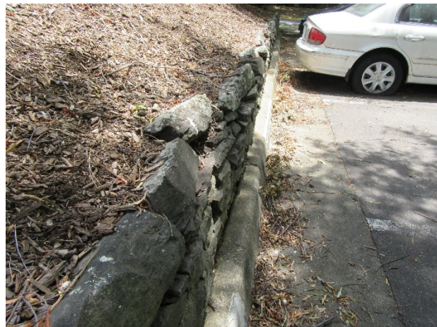
Stone displacement and minor bulging
