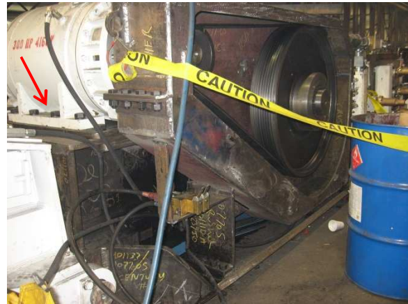
Figure 45. Motor Foot Mount Rigidly Bolted to Crusher Frame.
