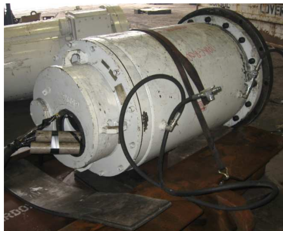
Figure 22. Motor On Test Viewed From Outboard End.
