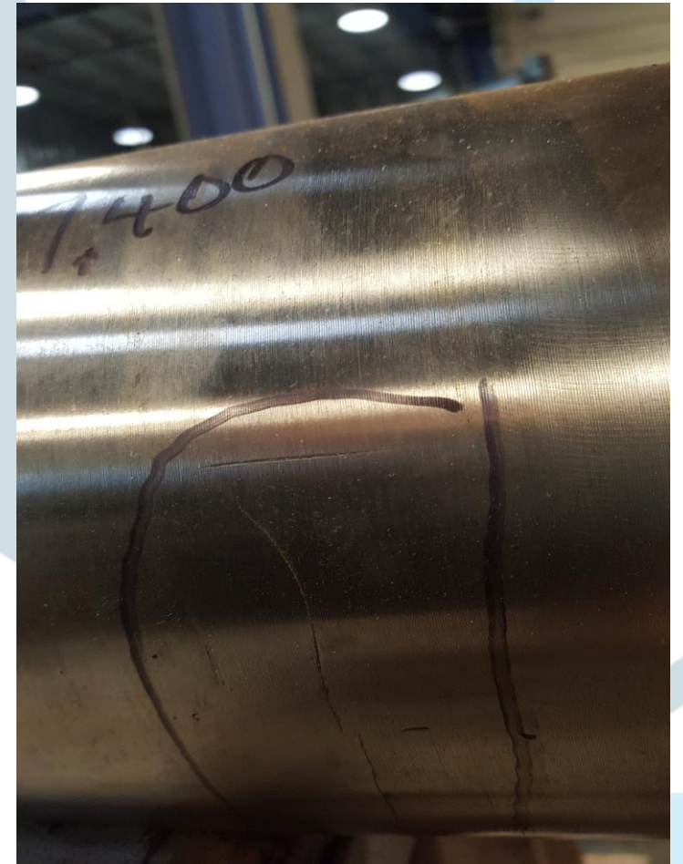
One of the Cracks
