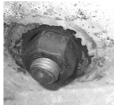
Figure 18. Motor Hold down Bolt, No Washer.
