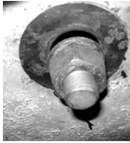
Figure 36. Motor Hold Down Bolt, Oversize Hole, No Washer.
