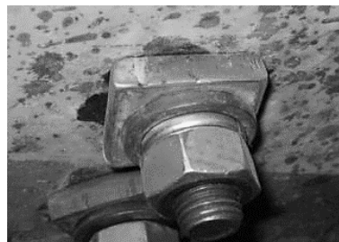
Figure 34. Fan A, Bearing Housing Hold Down Bolts.
