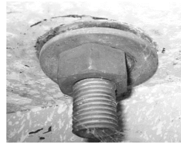
Figure 37. Fan A, Motor Hold Down Bolt With Deformed Flat Washer.
