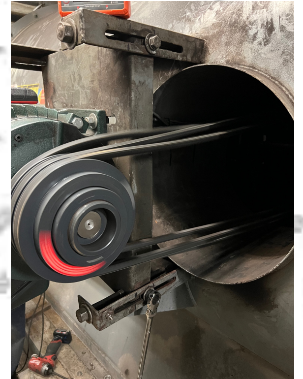
Air Handling Unit (Fan)
