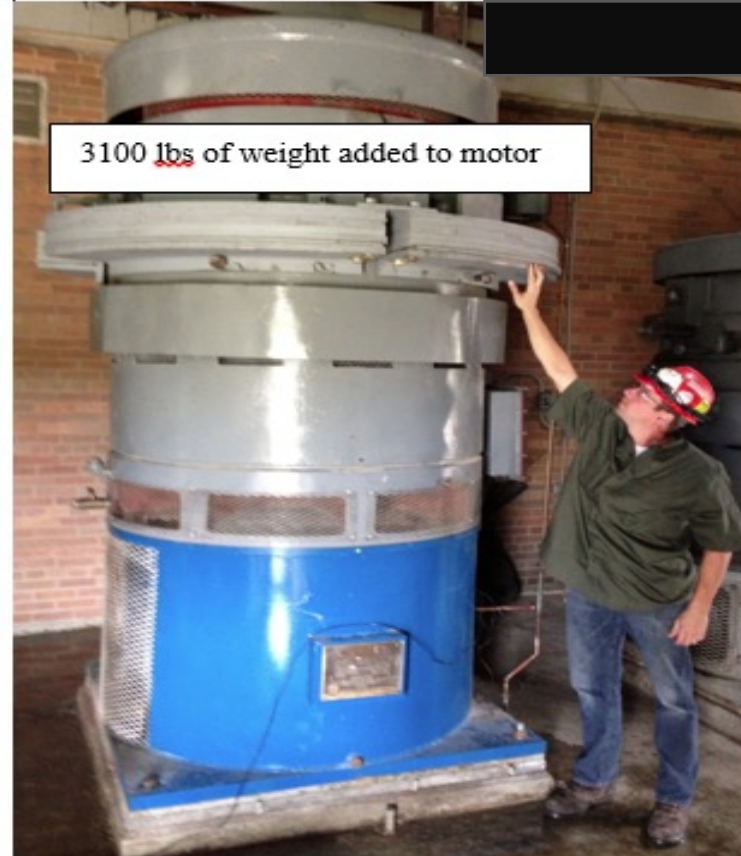
Vertical Pump with Mass added to reduce natural frequency
