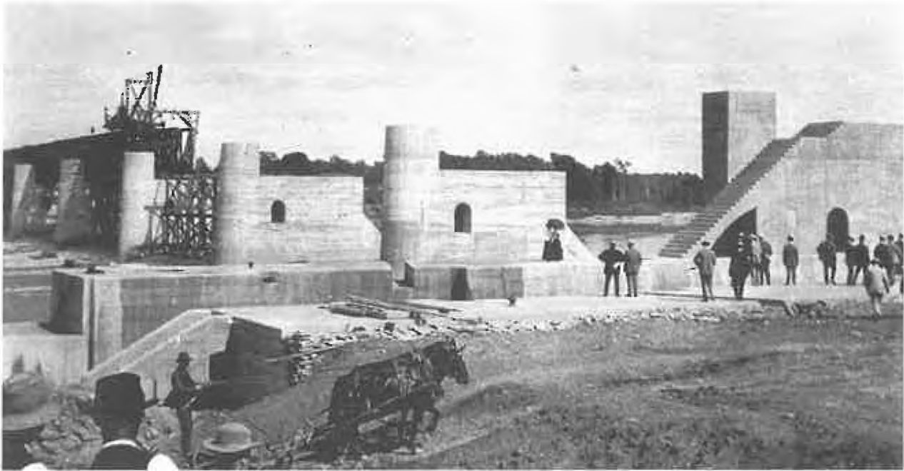
The seven bridge spans were erected in the summer of 1909 each with trusses 21ft wide x 126ft long.
