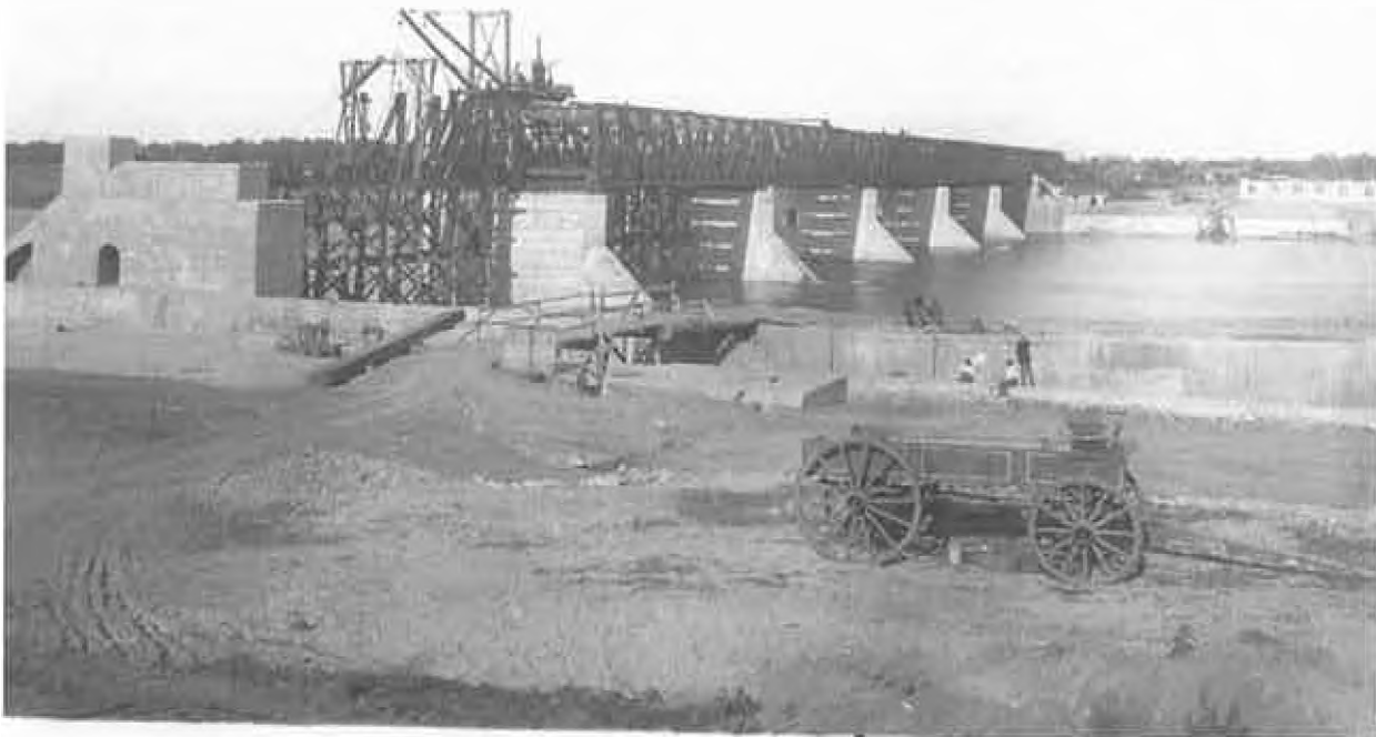
Steel frames being constructed that would contain the wooden roll curtains that formed the actual movable dam. Each curtain is made up of 50 Douglas Fir laths fitted into a heavy cast iron plate at the bottom. The frames weigh between 5-9 tons and are dropped to the concrete frame at the bottom of the dam. They can be adjusted according to river flows.
