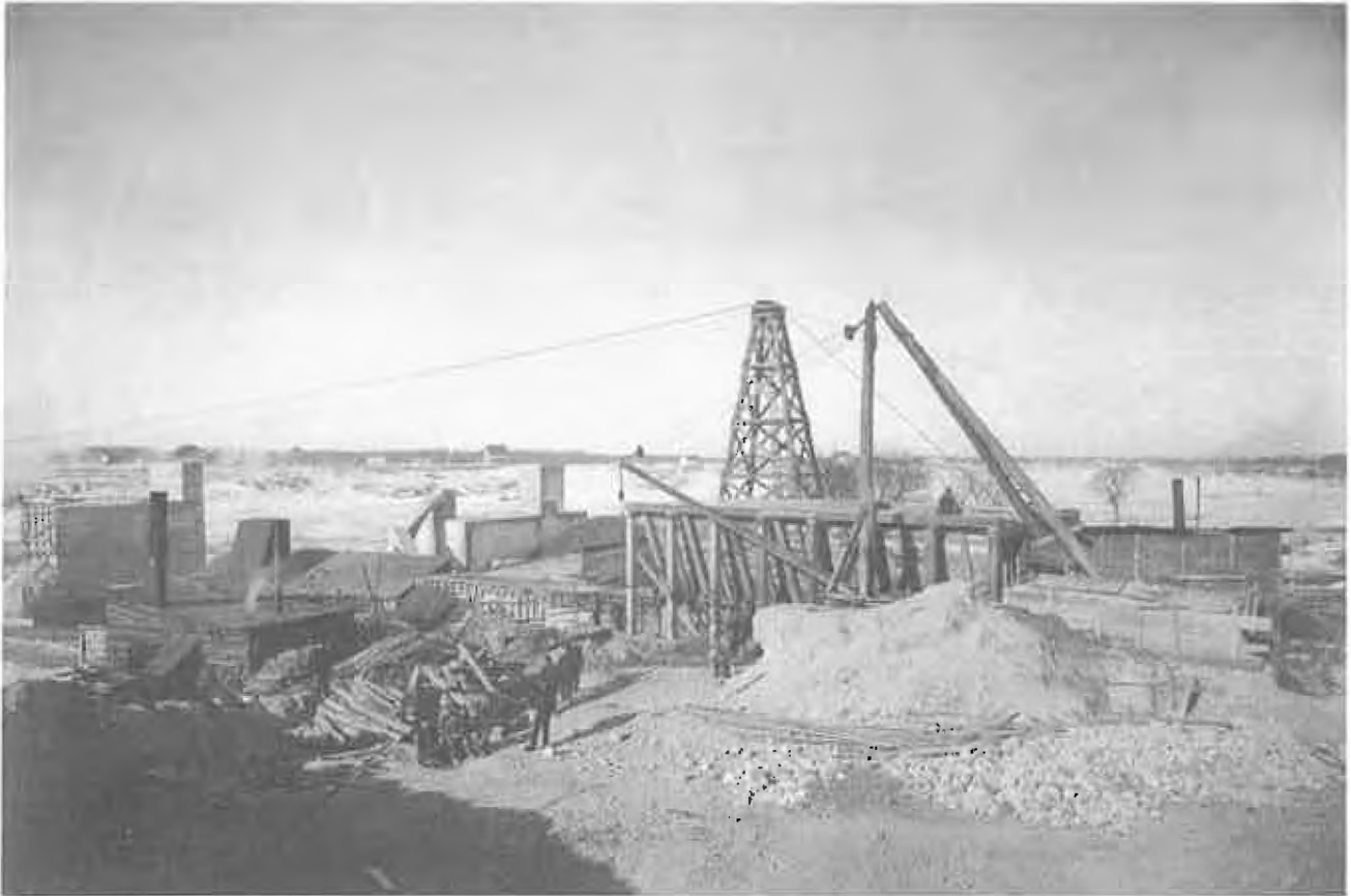
Most of the excavation work was accomplished in the winter months – provided the frost was not too severe
