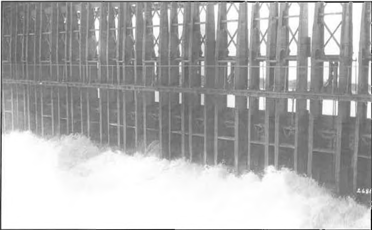
Steel frames weighing approximately 10 tons, are lowered into the water and the moveable wood lath gates are lowered into the frames to hold the water back.
