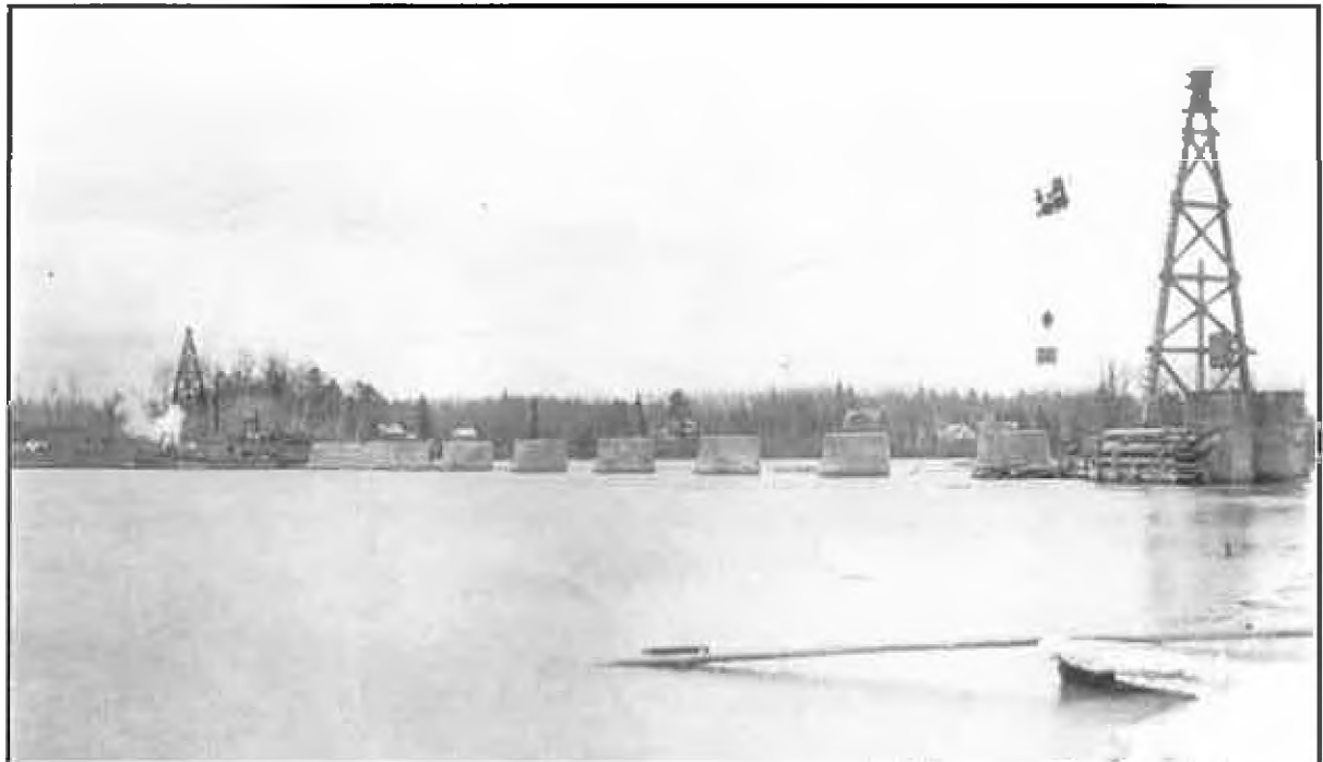
Cable tram ways were used to move concrete and other materials across the dam during construction
