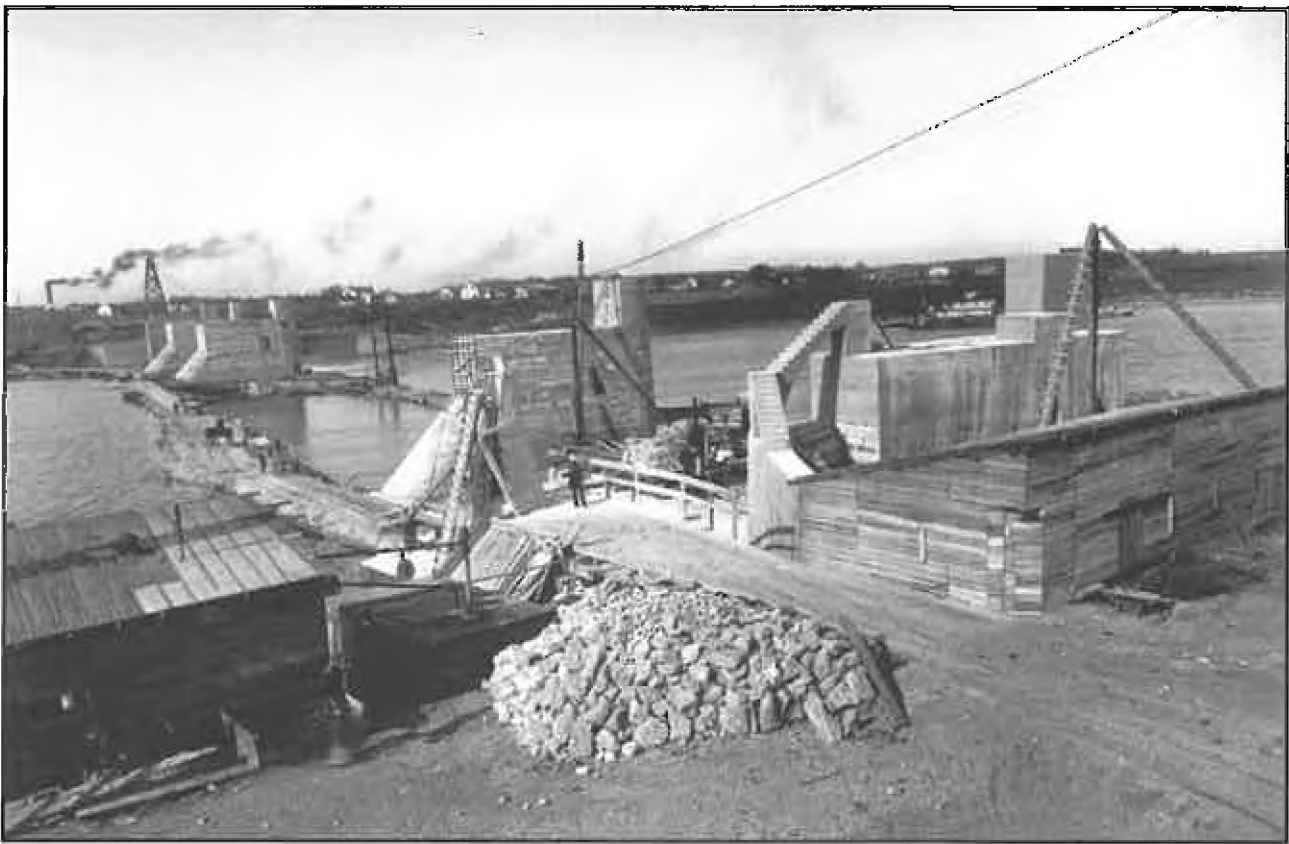
View of the main piers under construction. Note the temporary causeway / roadway located on either side of the row of piers and the tower and the cable mechanism used to carry huge buckets of concrete from the shoreline to the piers. (Manitoba Archives Photo.)
