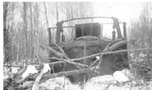
Bulldozing trees - there is a cutting blade on the bottom of the dozer blade to shear the trees off
