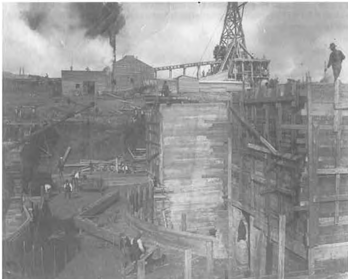
The building of the Lock, bridge piers and submerged dam began in 1905 and continued to 1908. Steel was supplied by Canada Foundry & Manitoba Bridge
