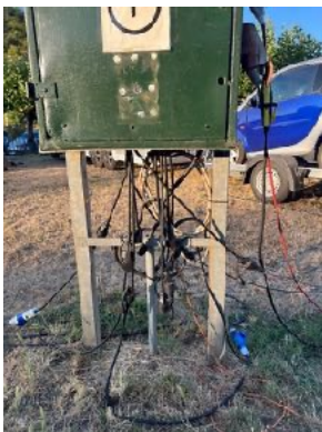
Electric post in Schweich, Germany – Photo by Amy Van Artsdalen
