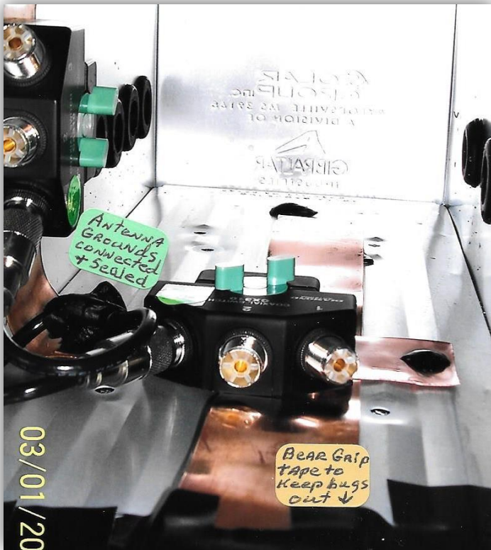
Photo #6 shows the coax seal which seals the polished/cleaned copper strap and brass screw ground connection and the bear tape is used to seal the crack at the bottom of the mailbox door while still allowing the door to open and close. This seals a large crack preventing "rain splash" and ants/spiders/critters from making their home in your outdoor mailbox and switchbox.
