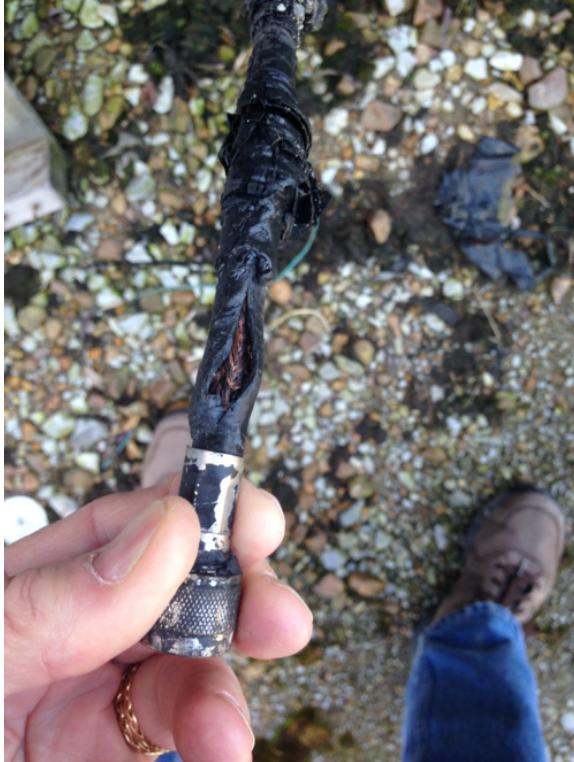
Break in coax on the old antenna Photo by Joe WA4OVO
