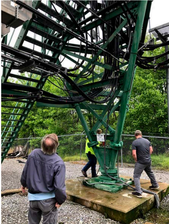
LOTS of cables!
