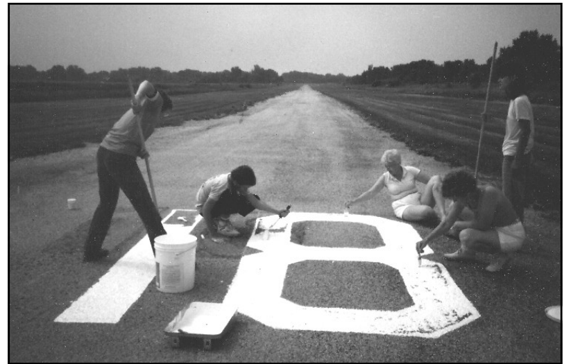
Chapter members paint runway numbers at Howell Airport, Crestwood, IL on June 20, 1987.
