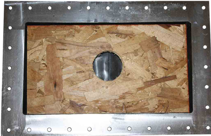
Wood board to prevent battery shorting against metal lid.
